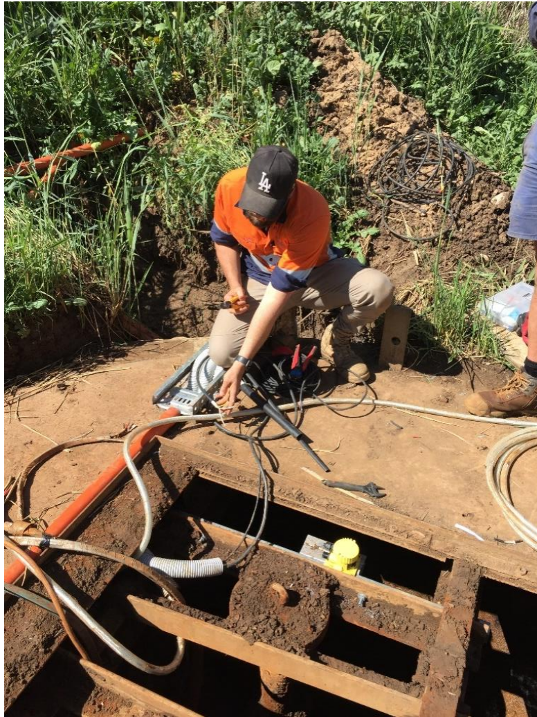
Photo: Installation of new pump at the Old River Pump Station Mendocorn.
