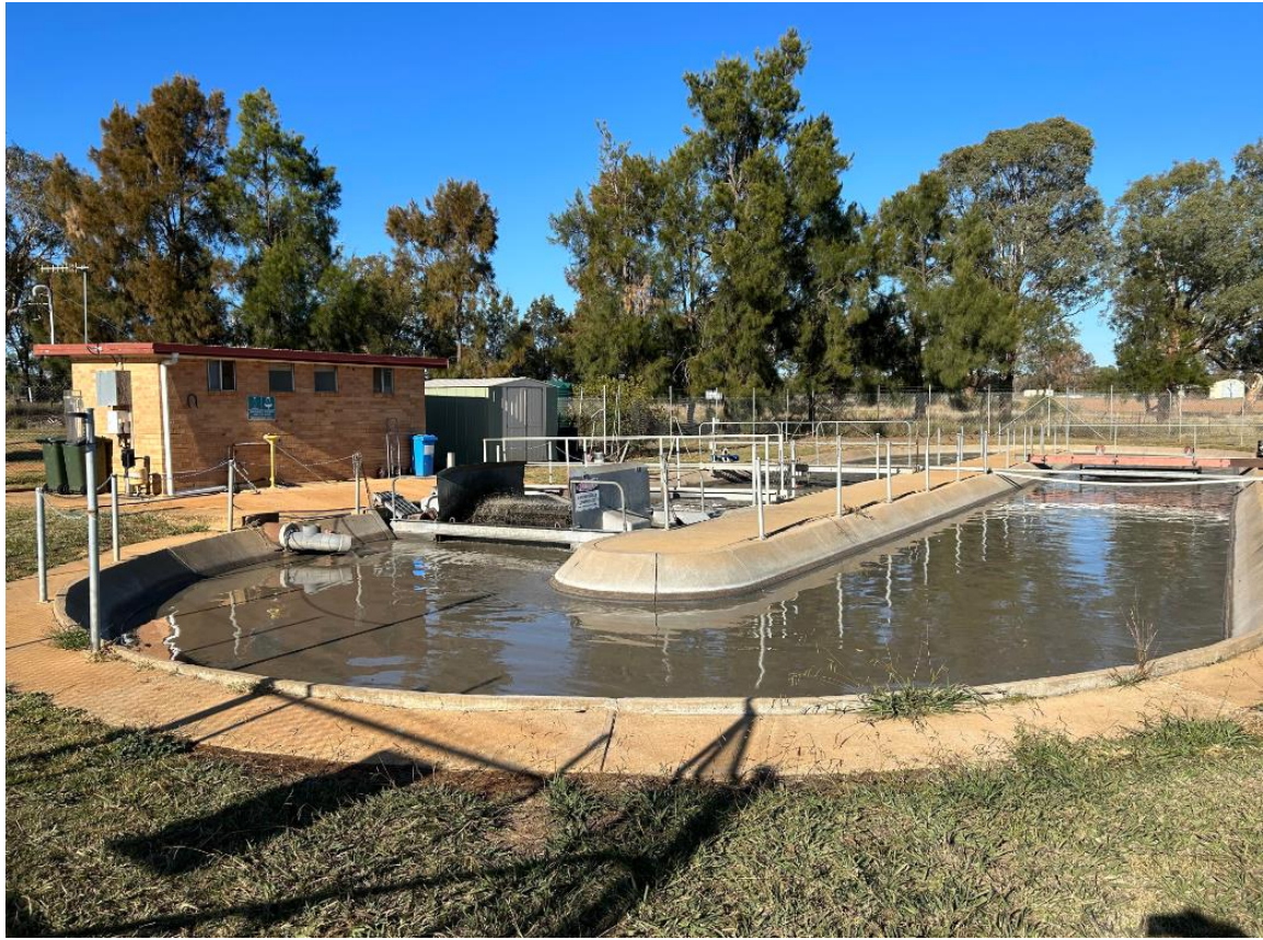
Photo: Dunedoo Wastewater Treatment Plant
