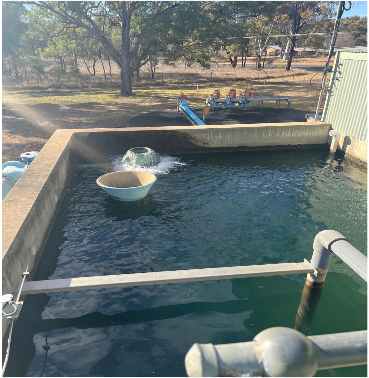
Photo: Coonabarabran Water Treatment Plant in action, settled water prior to filtration.
