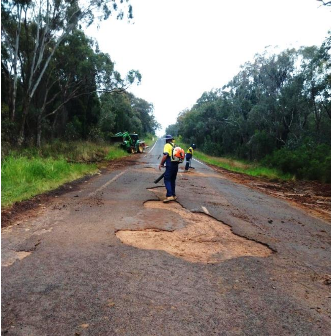
Photo: Pothole on the Castlereagh Highway, Dunedoo
