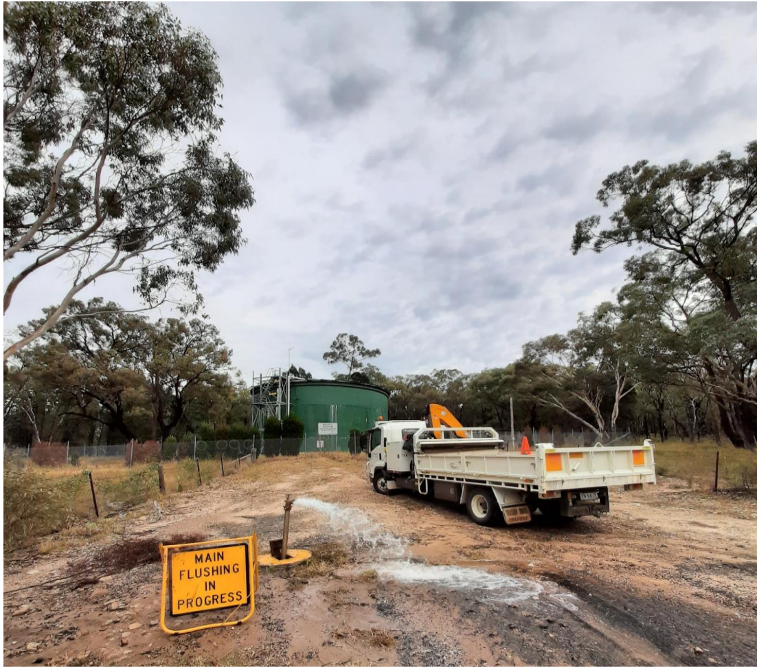
Image: Water from the new rising main being flushed to remove air and test for chlorine residual before it enters Martin street reservoir.
