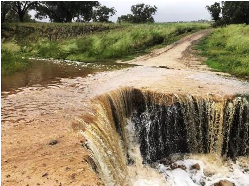
Photo Below – A road in Binnaway that has had extensive damaged caused by the rainfall.
