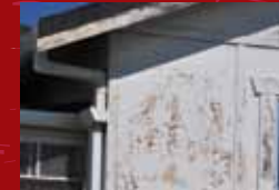
Exposed asbestos due to peeling paint
