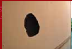
Holes in fibro walls
