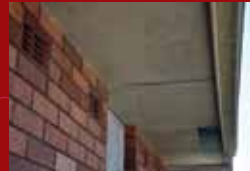
Unsecure eave joints
