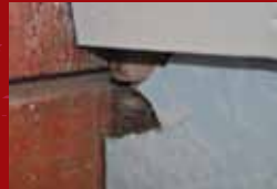
Damaged Tilux in bathrooms or laundries
