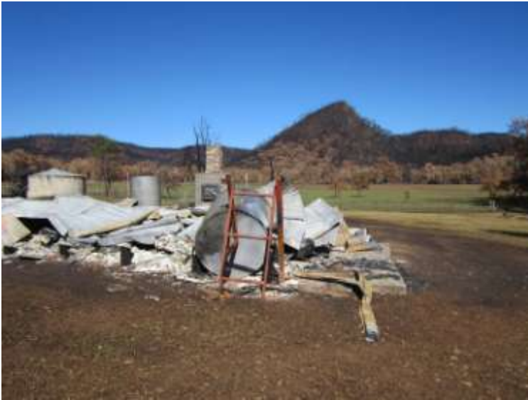
Figure 9 – Example of Fire Damaged property with Friable Asbestos and Soil to be removed
