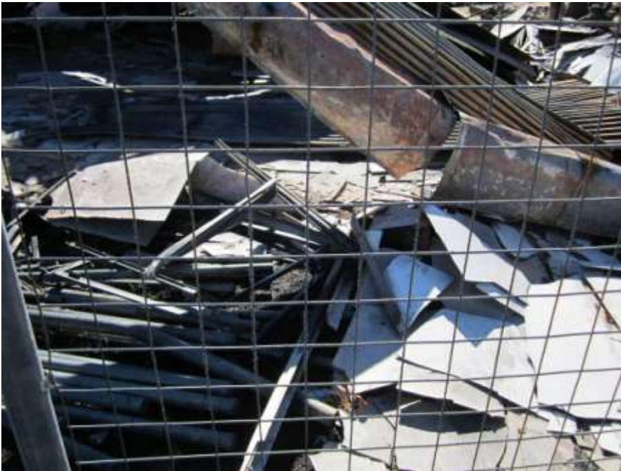
Figure 6 – Example of building collapsed due to structural fire damage. Collapsed ACM that has been reduced to a powder form or that can be crumbled or pulverised or reduced to a powder by hand pressure when dry is defined as friable asbestos.
