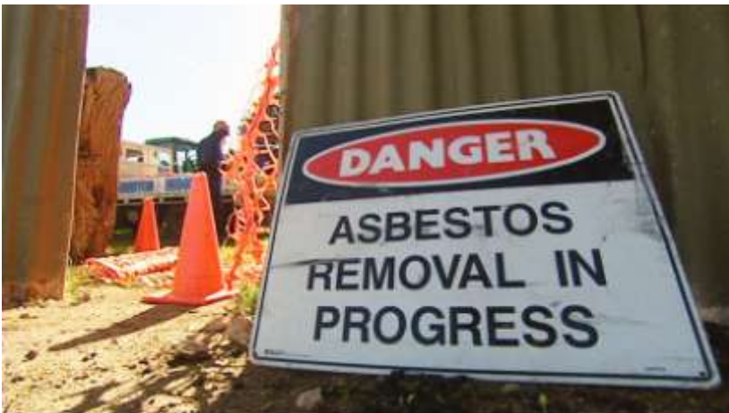
Figure 8 – Specified Asbestos Removal Signage
