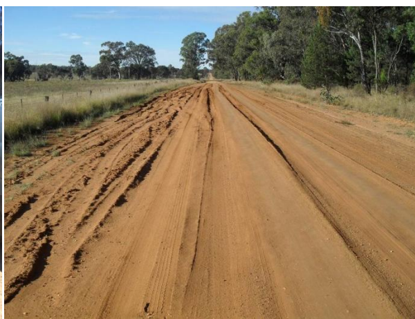
Condition 4: Very Poor (Unsealed)
