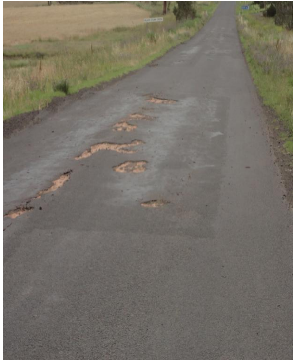
Condition 4: Very Poor (Sealed)
