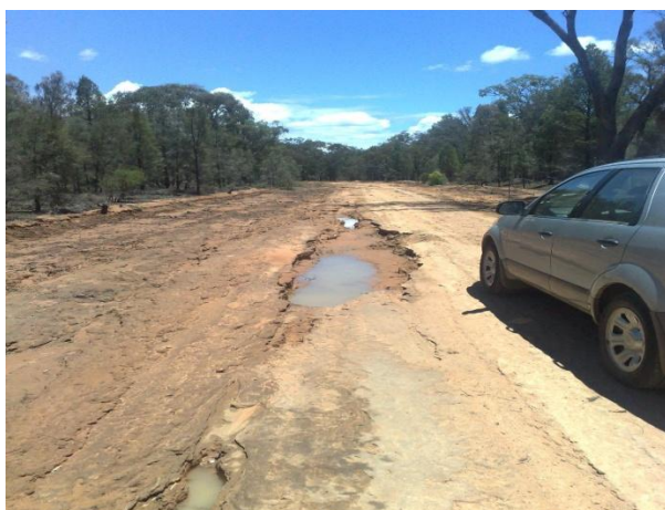
Condition 3: Poor (Unsealed)
