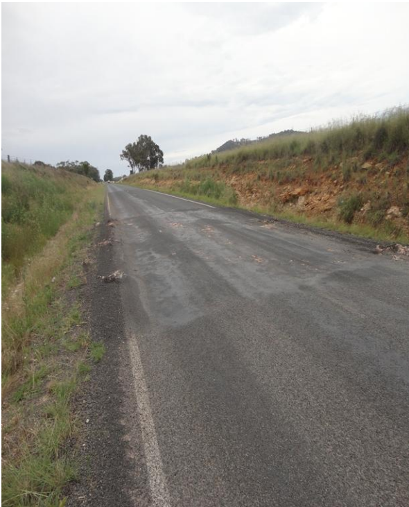
Condition 3: Poor (Sealed)
