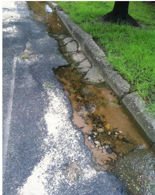
Condition 4: Very Poor
